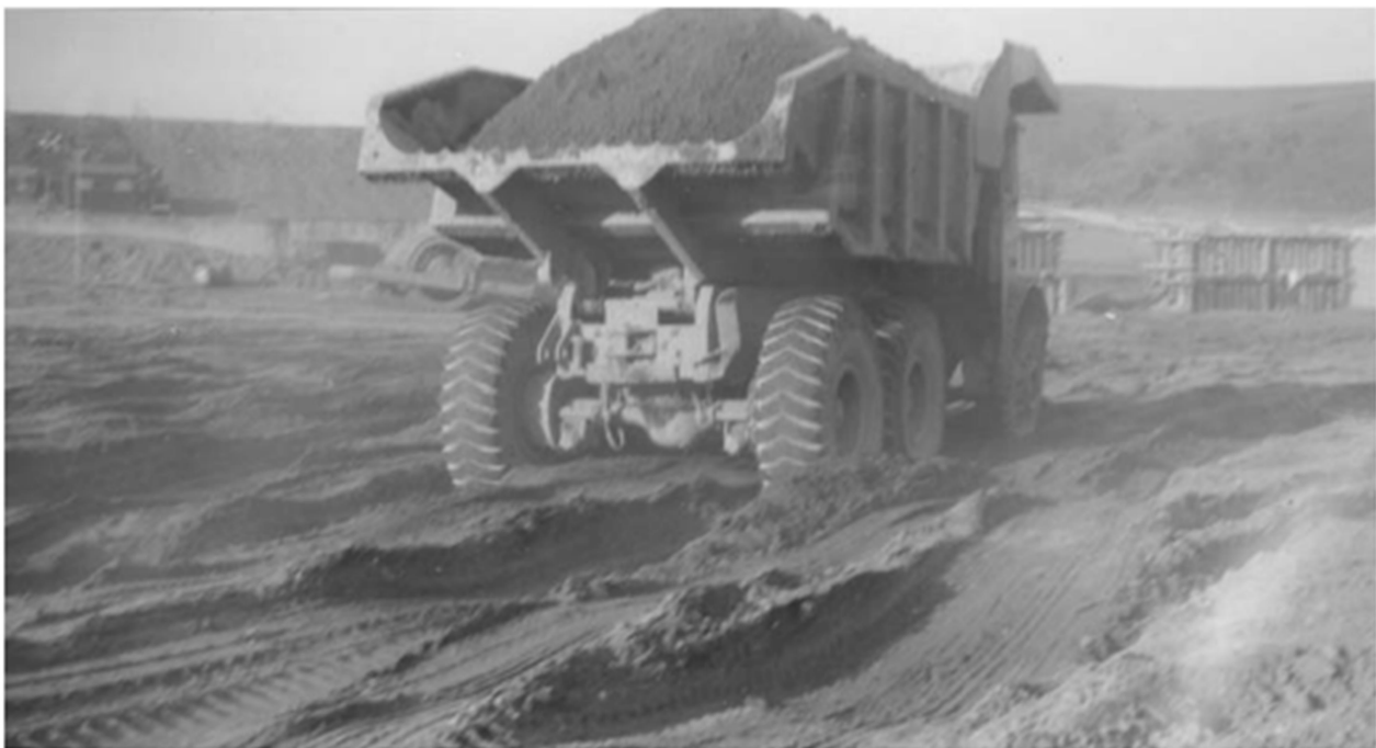
Plate 4b. A badly rutted formation, probably due to excessive moisture content of the fill
