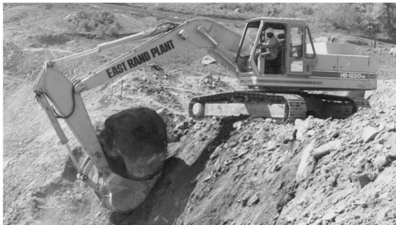
Plate 3b. A Kato 162 kW tracked excavator, with 1.6 m 3 bucket. ACP Holdings, Leicester, UK
