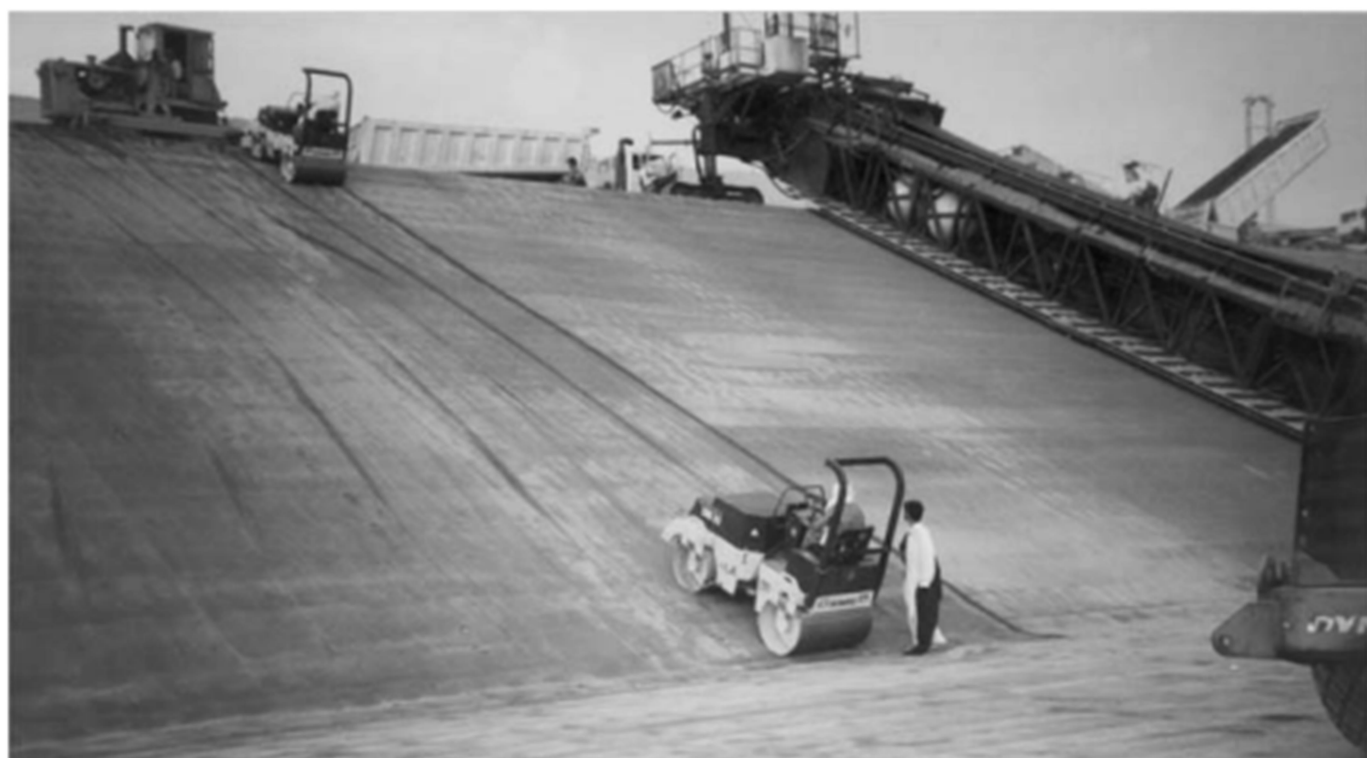
Plate 4a. Rollers compacting side slopes of power channel; filter layers and concrete to follow. Ghazi Barotha Hydropower project, Pakistan 1999
