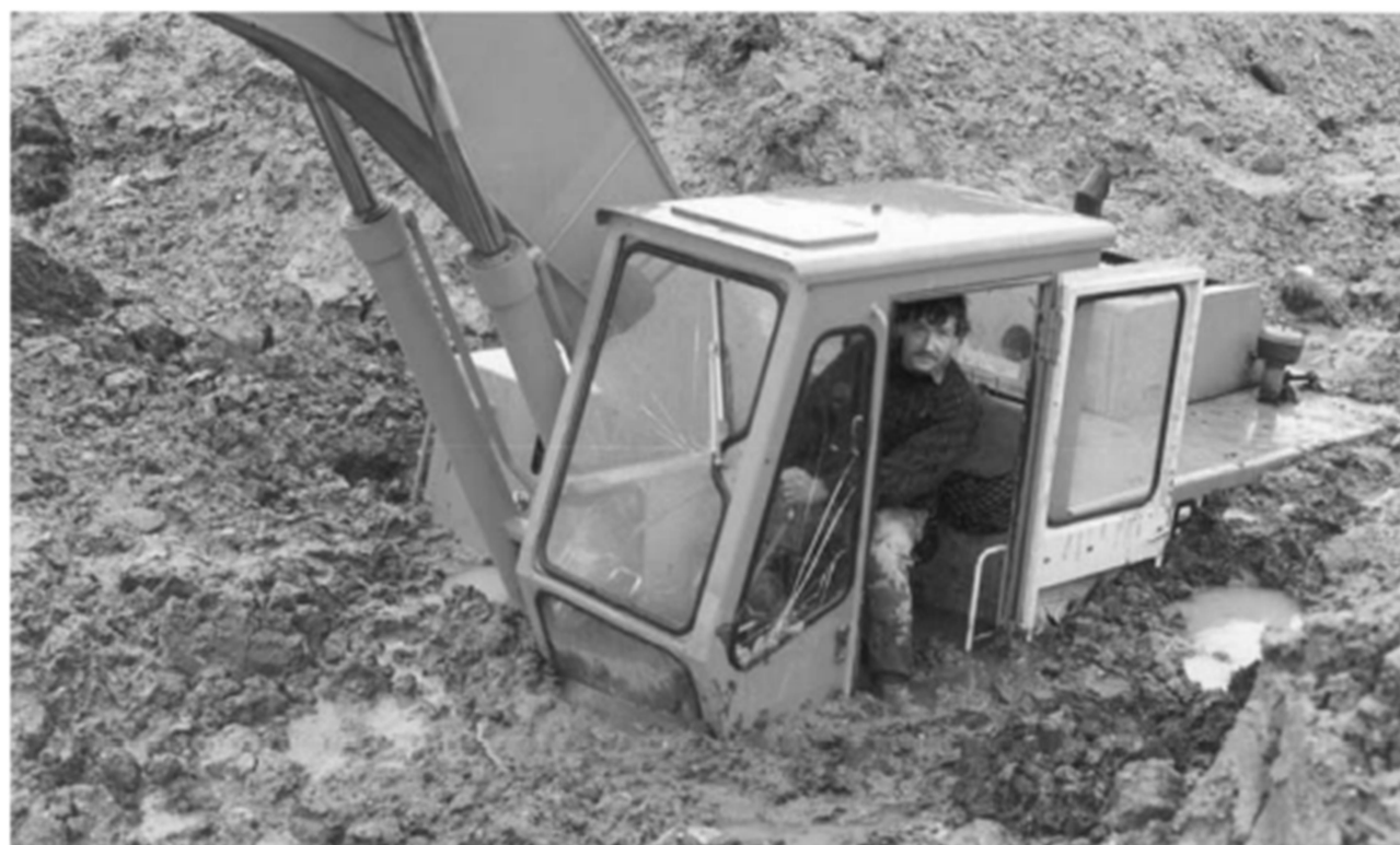
Plate 5b. It can be easier to get out of this sort of trouble than to decide whether the conditions 'could not reasonably have been foreseen by an experienced contractor' under Clause 12 of the ICE conditions
