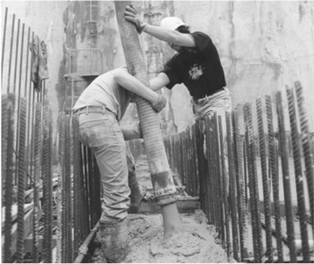
Plate 14a. The typical fluidity of pumped concrete; but it still needs vibrating in place
