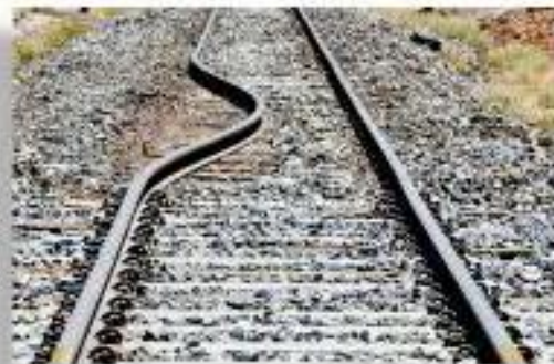
Buckling of rails Due to a heatwave in country Victoria
